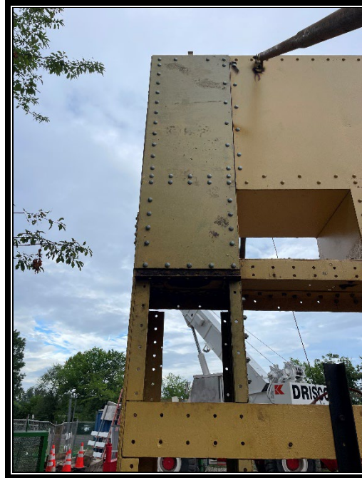
Figure 2: Additional repair area on East Tide Gate.
