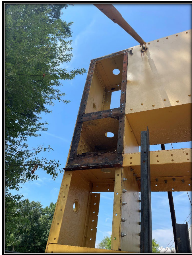
Figure:1 Additional repair area on East Tide Gate.
