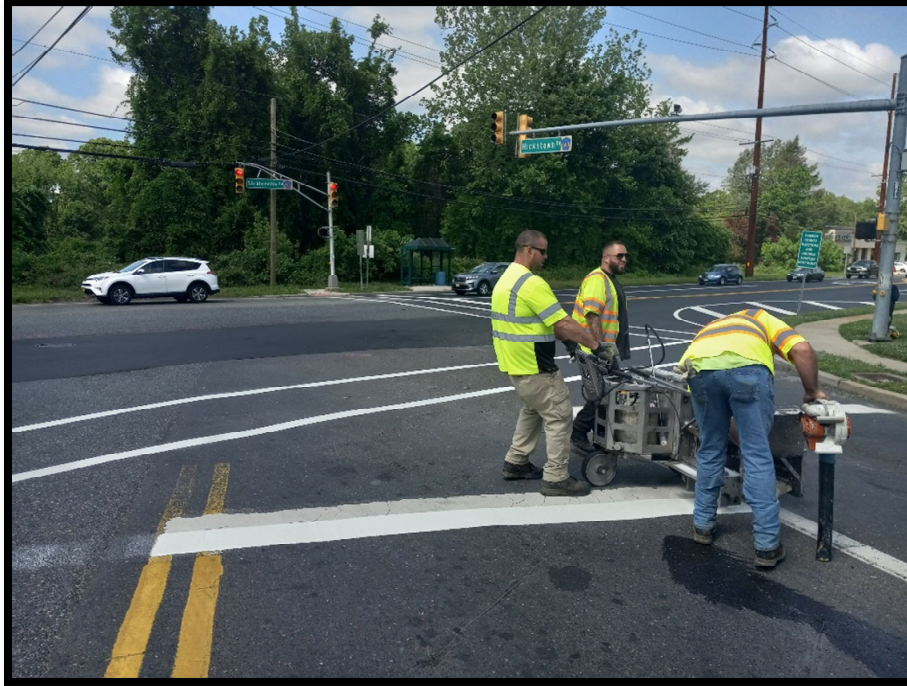
Photograph 2 - Typical Stop Bars and Standard Cross Walk Striping being installed at the intersection of Sicklerville Road (CR 705) and Hickstown Road.
