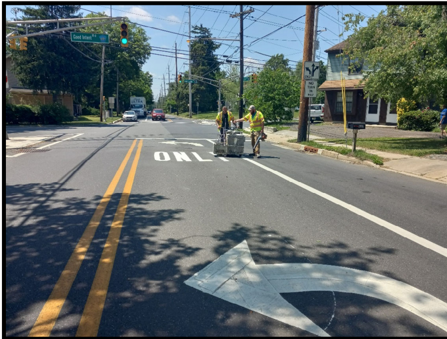
Photograph 3 – Turn Arrows and “ONLY” being installed on Almonesson Road (CR 706) at the Lower Landing Road intersection.
