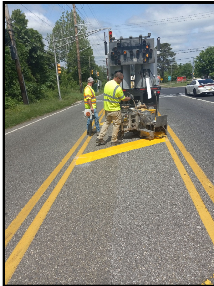
Photograph 1 – Typical 24" Yellow Thermoplastic Gore Striping being installed on Sicklerville Road (CR 705) near the intersection of Hickstown Road.
