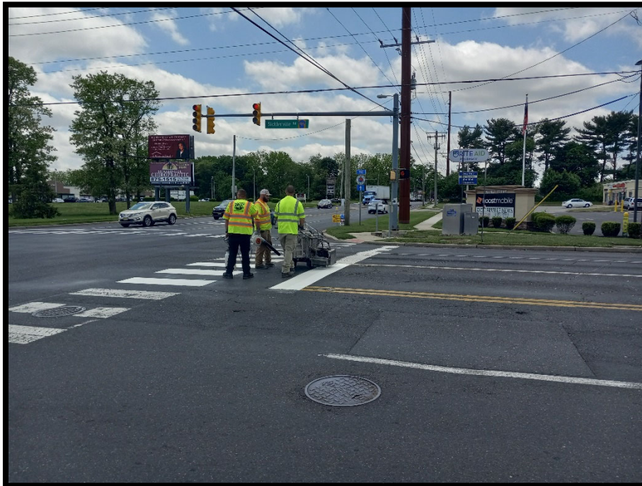
Photograph 3 – Piano Key Cross Walk and Stop Bar being installed on Sicklerville Road (CR 705).
