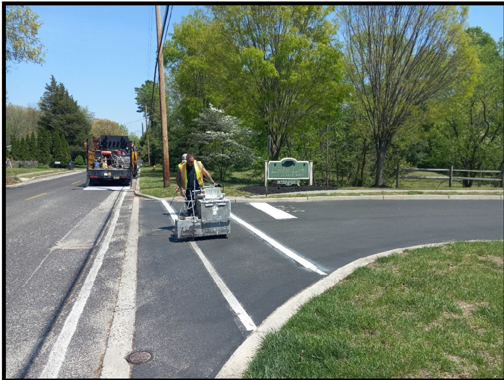
Photograph 1 – 24" White Thermoplastic Stop Bar and Standard Cross Walk Striping being installed along Norcross Road near Linden Lake Senior Apartments.
