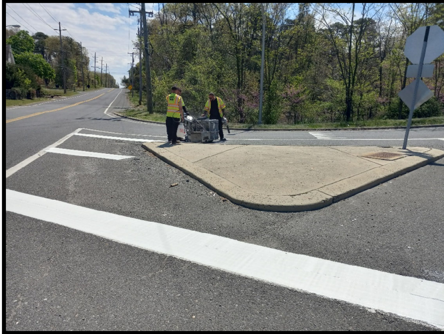
Photograph 2 – Typical White Gore Striping being installed at the Egg Harbor Road (CR 702) intersection with United States Avenue.
