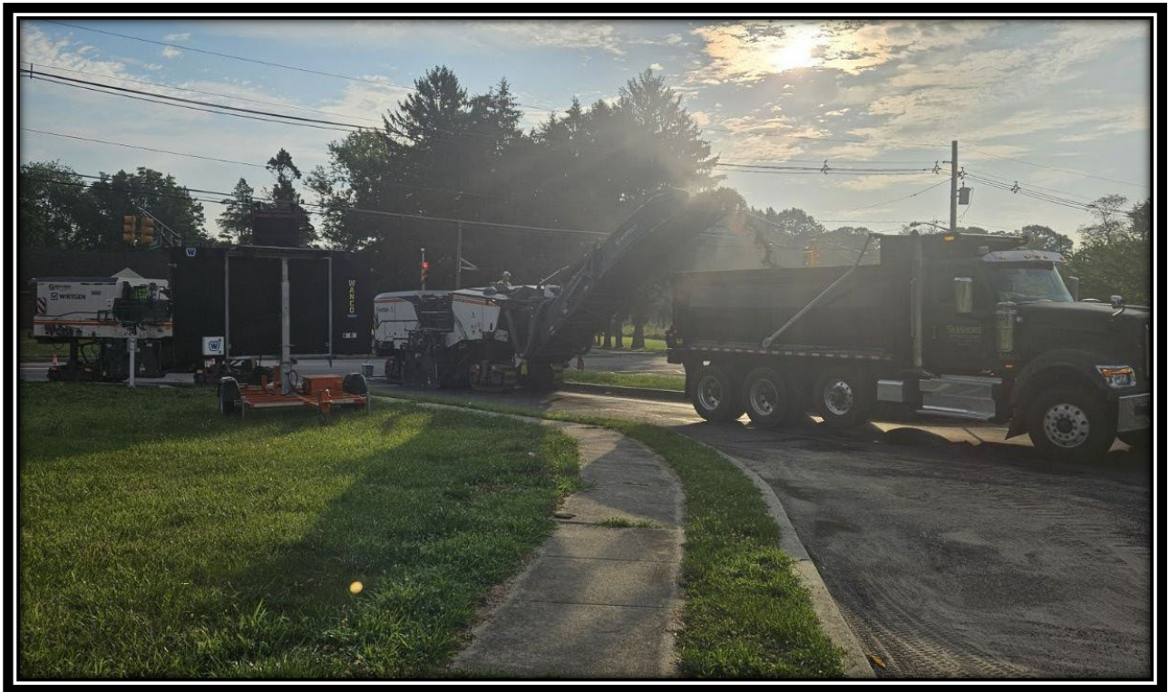
Figure: 1 – 2” Milling of southbound lane at the intersection with Chews Landing Road
