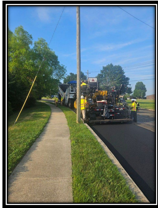
Figure: 2 – Installation of 2” thick HMA 12.5M64 Surface Course along the southbound lane between Chews Landing Road and Golfview Drive
