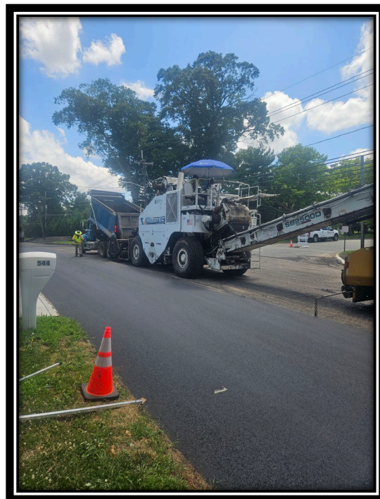
Figure: 3 – Installation of 2” thick HMA 12.5M64 Surface Course along the southbound lane at the intersection with Golfview Drive
