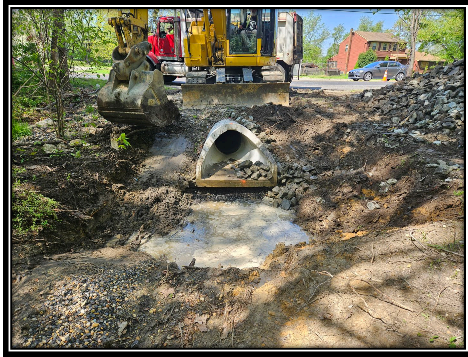
Figure: 2 – Installation of scour hole and slope stabilization at concrete flared end section between Tall Oaks Drive and Mt. Pleasant Road
