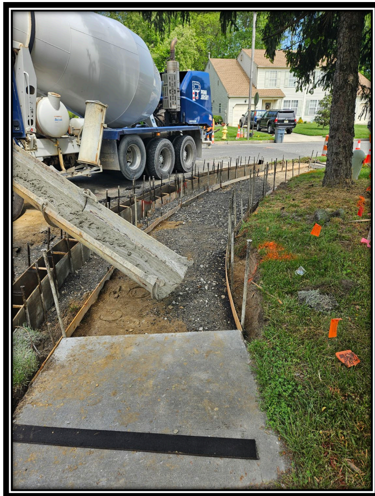
Figure: 1 – Installation of concrete sidewalk and curb along the northbound lane at the intersection with Woodmill Drive
