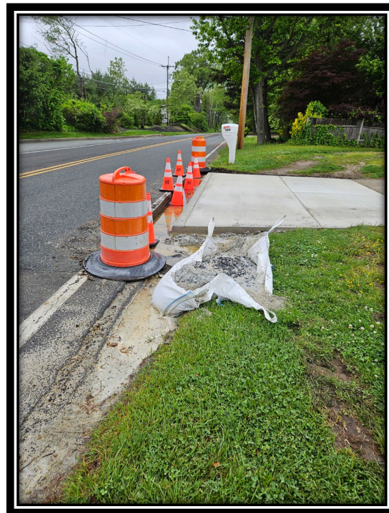
Figure: 3 – Installation of 6” Thick, reinforced concrete driveway apron along the northbound lane between Hider Lane and Golfview Drive
