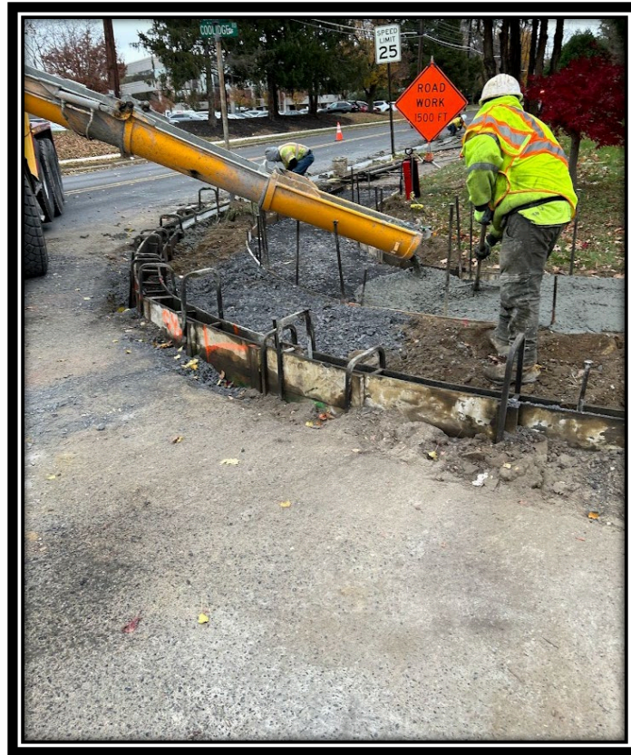
Figure: 2 – Installation of concrete curb, sidewalk, and ADA ramp along the eastbound lane at the intersection with Coolidge Road
