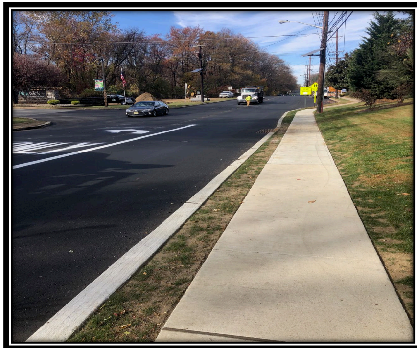
Figure: 3 – Installation of thermoplastic traffic striping and markings between the County Border and King's Highway
