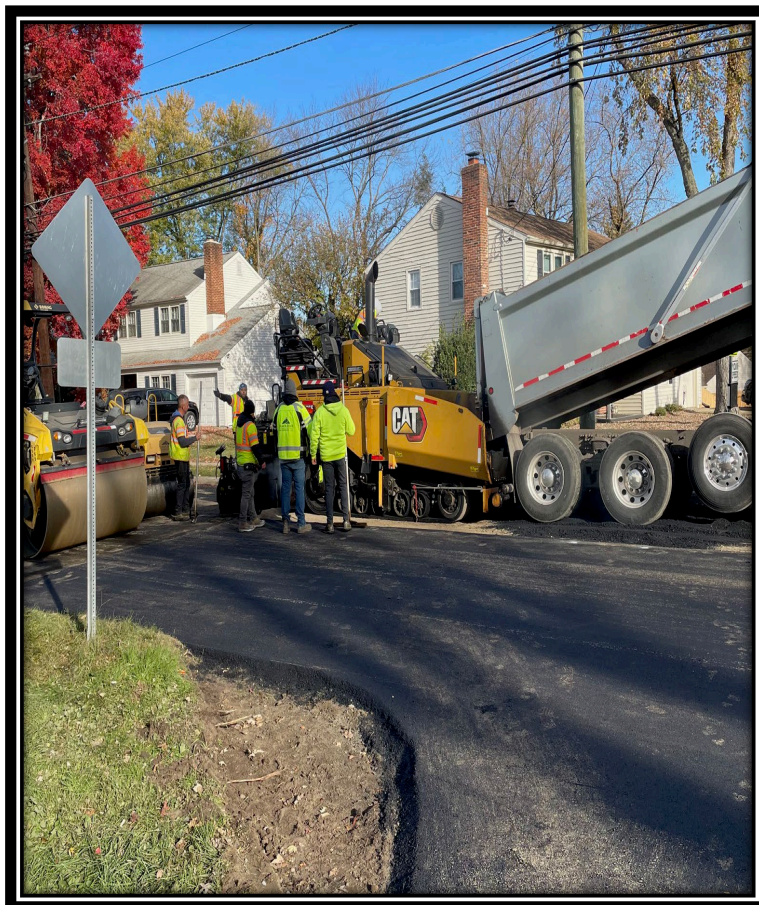
Figure: 1 – Installation of HMA 19M64 base course in the westbound lane between Millstream Drive and King’s Highway
