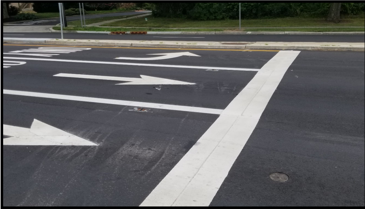
Photograph 3 – Raised Pavement Markers installed along Greentree Road near the Springdale Road intersection.
