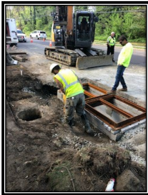
Figure: 1 – Installation of Double E Inlet along the eastbound lane between DaCosta Drive and Kings Highway
