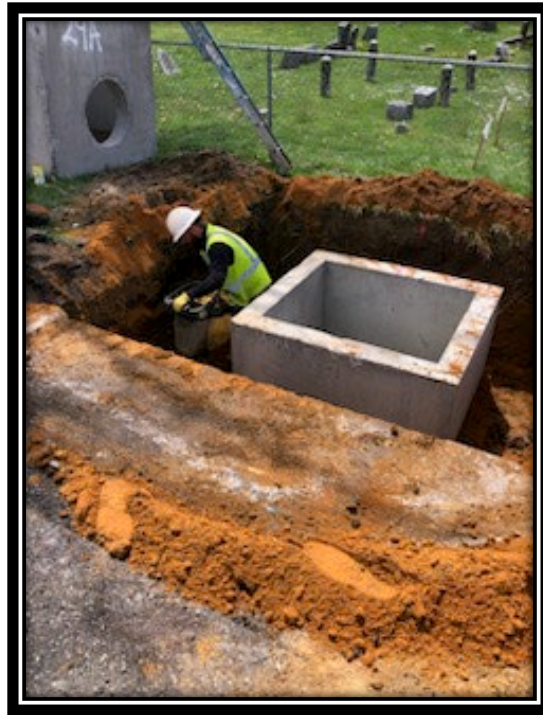
Figure: 2 – Installation of B Inlet along the eastbound lane between Kings Highway and Friendship Lane
