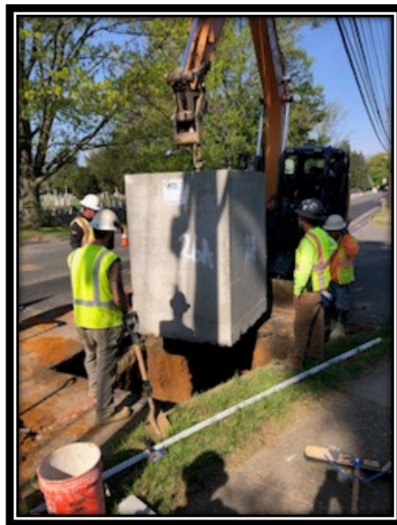
Figure: 3 – Installation of E Inlet along the westbound lane between Kings Highway and Friendship Lane
