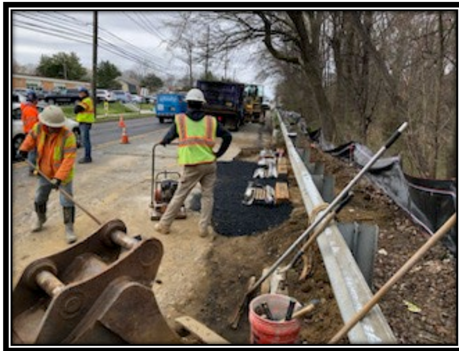
Figure: 3 – HMA restoration in front of newly installed Type Double B and B Inlets the eastbound lane between Kings Croft Drive and the County Border
