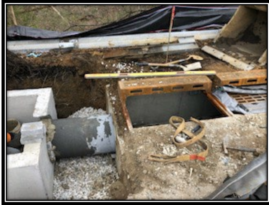
Figure: 2 – Installation of Type Double B Inlet along the eastbound lane between Kings Croft Drive and the County Border
