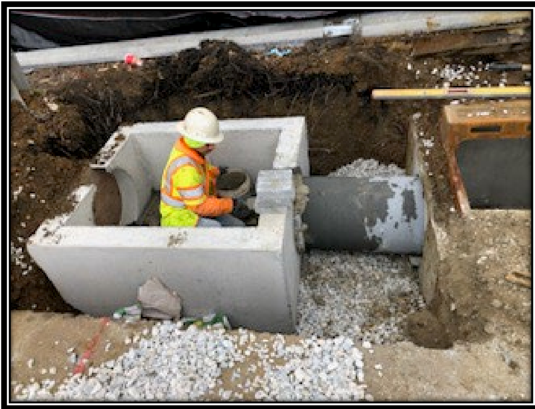
Figure: 1 – Installation of Type B Inlet along the eastbound lane between Kings Croft Drive and the County Border
