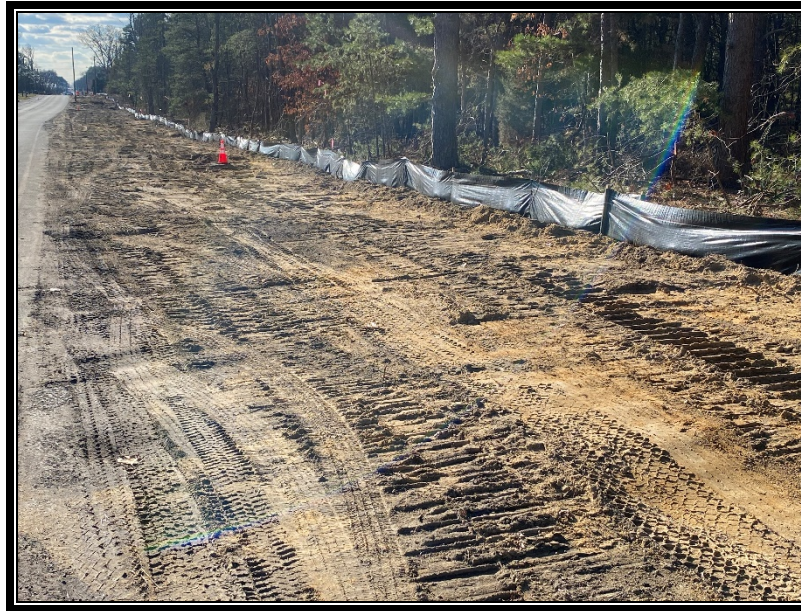
Figure 2: P&A Construction continues to install the silt fence along the limit of disturbance.
