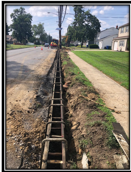
Figure: 3 – Forming of concrete curb along the westbound lane between Millstream Drive and Madison Avenue
