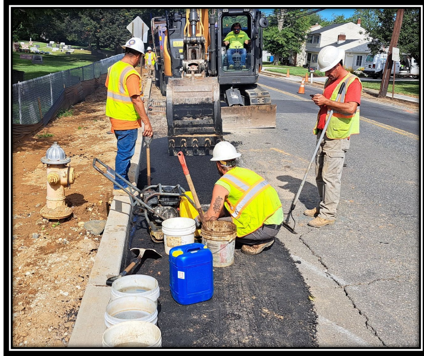
Figure: 2 – Road widening and concrete curb HMA trench restoration along the eastbound lane between Millstream Drive and King’s Highway
