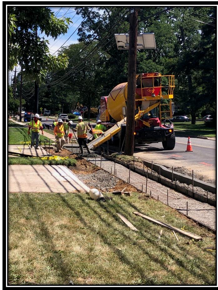
Figure: 1 – Installation of reinforced concrete driveway apron, sidewalk and curb along the westbound lane between Friendship Drive and Millstream Drive
