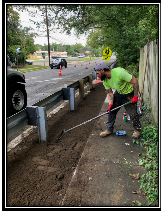
Figure: 2 – Topsoil, seed and fertilizer restoration around newly installed ADA ramp, concrete sidewalk and guide rail along the eastbound lane between DaCosta Drive and the County line
