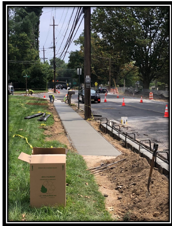
Figure: 3 – Installation of concrete sidewalk and curb along the westbound lane at the intersection with Friendship Drive
