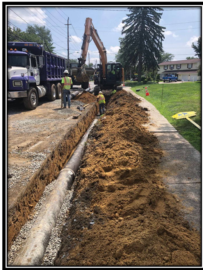
Figure: 1 – Installation of 12” DIP storm sewer along the eastbound lane between Roosevelt Boulevard and Cleveland Avenue
