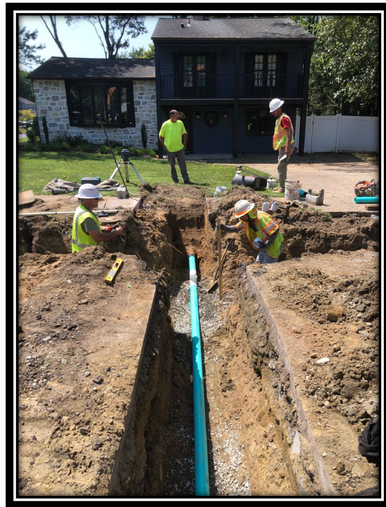
Figure: 3 – Relocation of a residential sanitary sewer lateral along the eastbound lane between Roosevelt Drive and Cleveland Avenue
