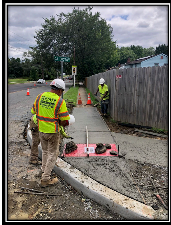
Figure: 2 – Installation of ADA ramp and concrete sidewalk along the eastbound lane at the intersection with DaCosta Drive
