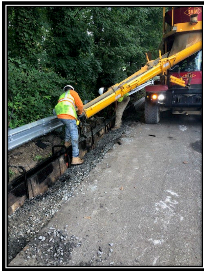
Figure: 1 – Installation of concrete vertical curb along the eastbound lane between DaCosta Drive and the County Border
