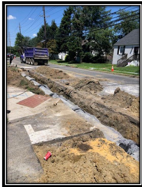
Figure: 3 – Installation of 18” RCP storm sewer along the westbound lane between Lincoln Avenue and Roosevelt Drive
