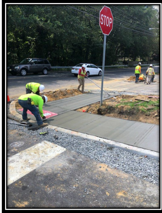
Figure: 2 – Installation of ADA ramp and concrete sidewalk along the westbound lane in front of the Thomas Paine Elementary School
