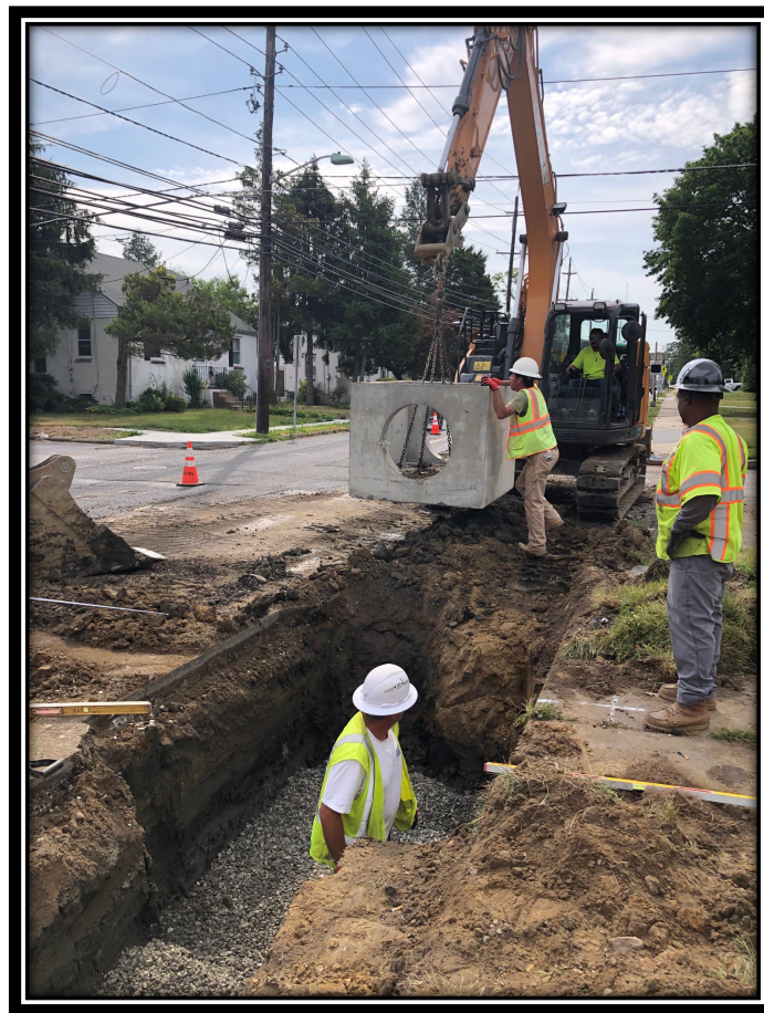
Figure: 1 – Installation of Type B inlet along the eastbound lane at the intersection with Lincoln Avenue
