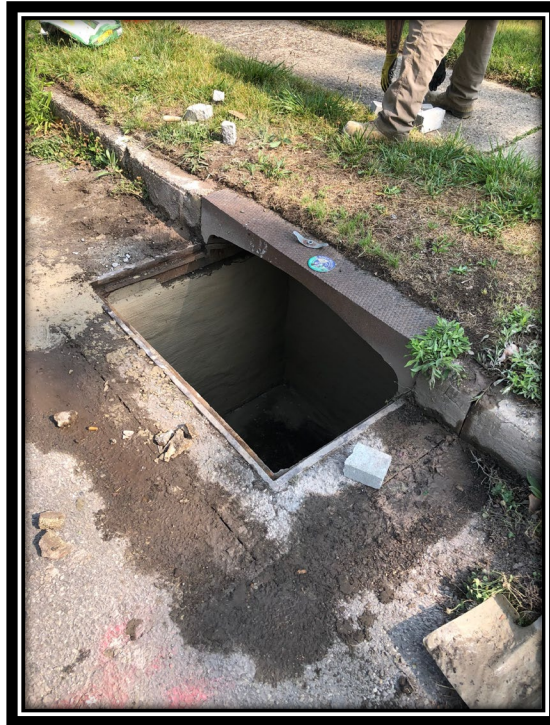
Figure: 2 – Reconstruction of existing B inlet along the westbound lane between Wilson Road and Lincoln Avenue
