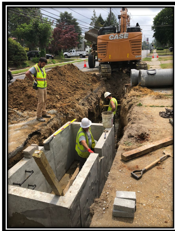
Figure: 3 – Installation of Type Double B inlet along the eastbound lane at the between Wilson Road and Lincoln Avenue
