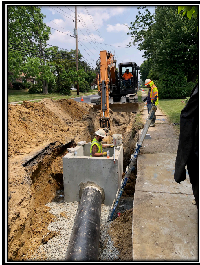
Figure: 1 – Installation of Type B inlet and 18” DIP along the eastbound lane between Wilson Road and Lincoln Avenue
