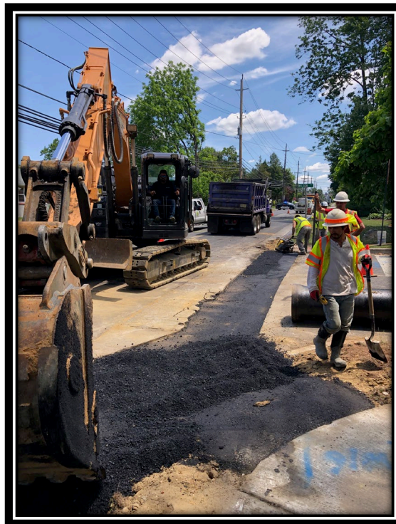
Figure: 3 – Roadway restoration of newly installed 18” DIP and 18” RCP storm sewer trench between Wilson Road and Lincoln Avenue
