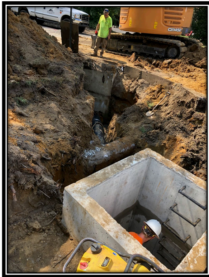
Figure: 1 – Installation of Type B Inlet, 6’-8.5’ Deep, at the intersection with Washington Avenue
