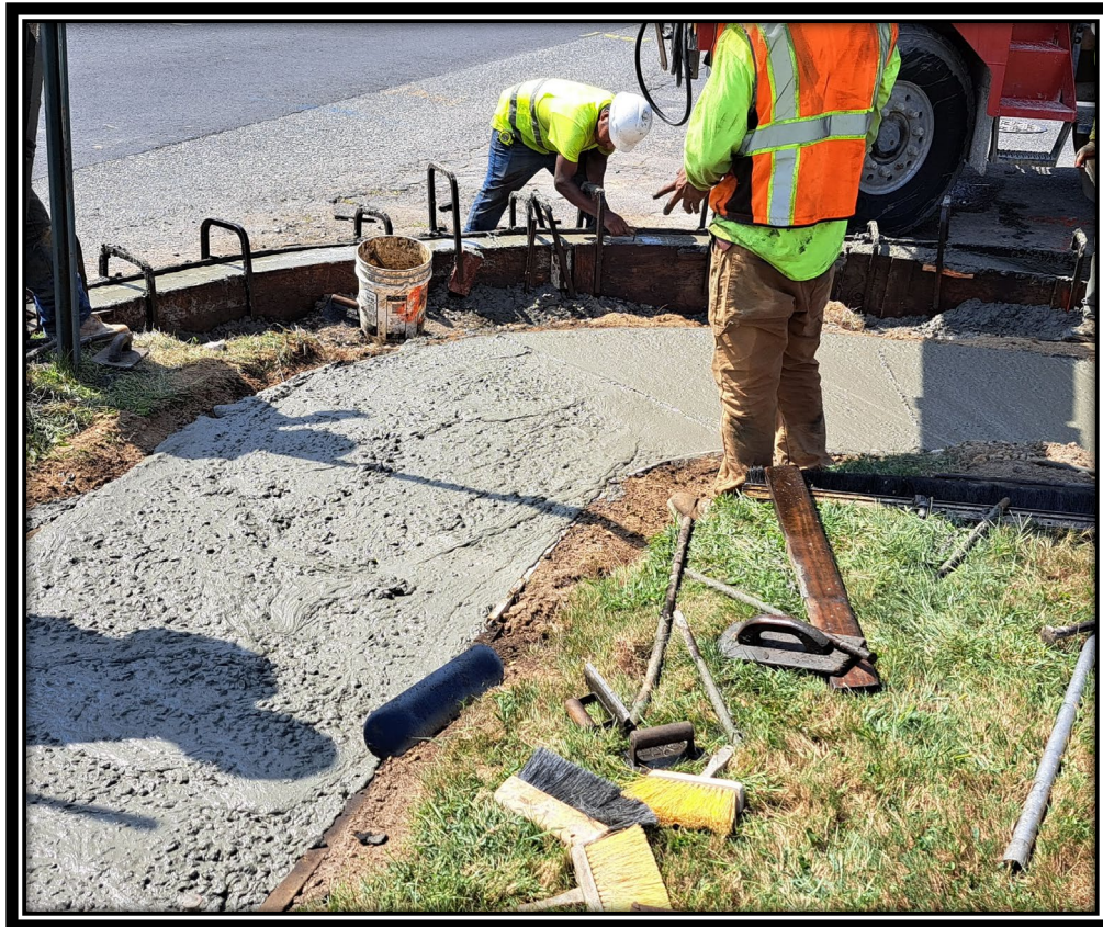
Figure: 2 – Installation of concrete curb and sidewalk along the eastbound lane at the intersection with Cleveland Avenue
