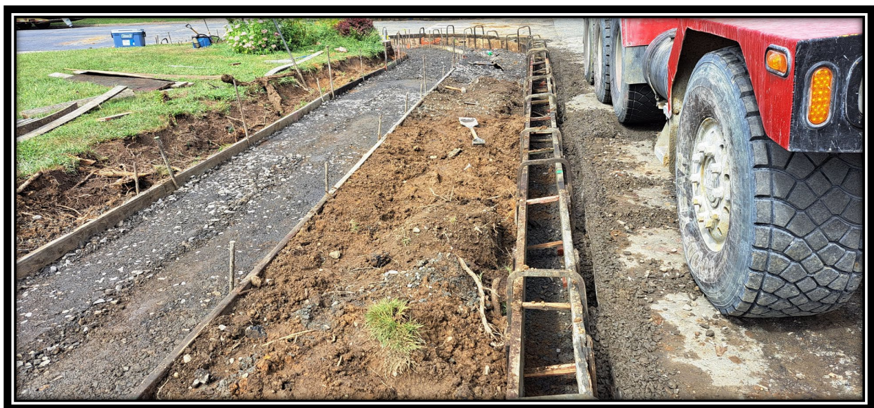
Figure: 3 – Forming of concrete curb and sidewalk along the eastbound lane approaching the intersection with Cleveland Avenue
