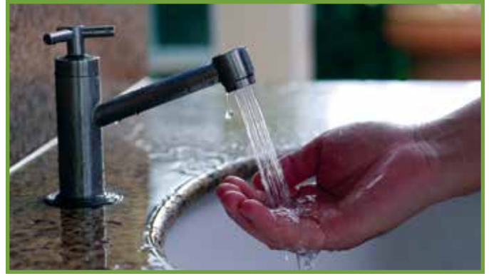
Install a high efficiency faucet aerator
