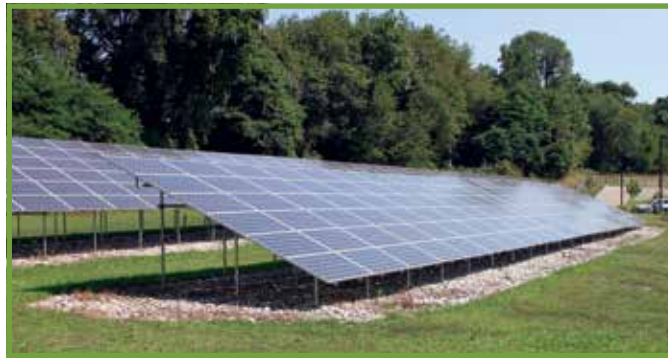
Solar array at the Camden County Lakeland Complex Gloucester Township – Source: Camden County
