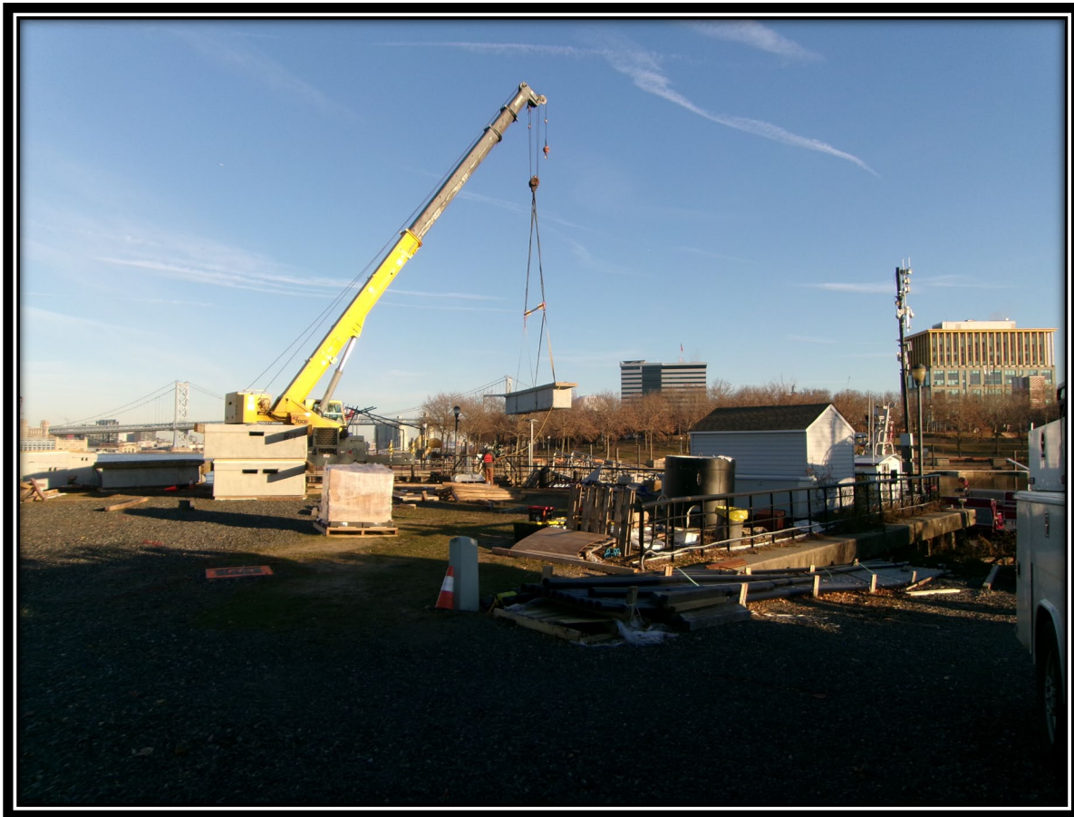
Figure: 1 – Moving of concrete floating finger pier section to be installed at the main pier
