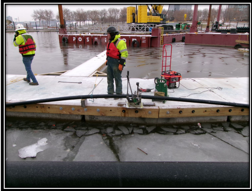
Figure: 2 – Installation of 3” PVC fire service along southern end of the main floating dock
