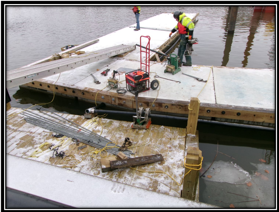
Figure: 3 – Installation of 3” PVC fire service along southern end of the main floating dock and connection to the main pier
