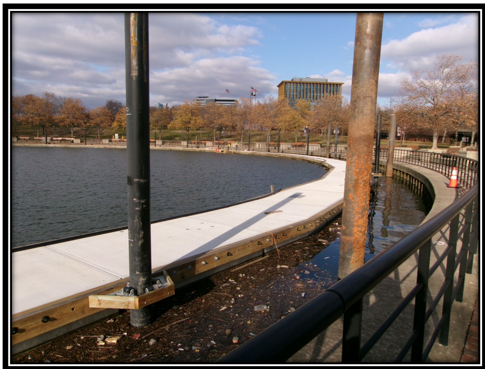
Figure: 3 – Installation of 2” PVC water service at the southern and eastern ends of the marina
