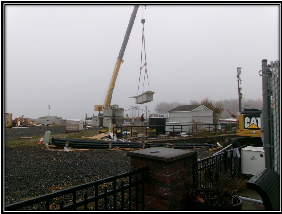
Figure: 1 – Moving of concrete floating finger piers to be installed at the far northern end of the marina
