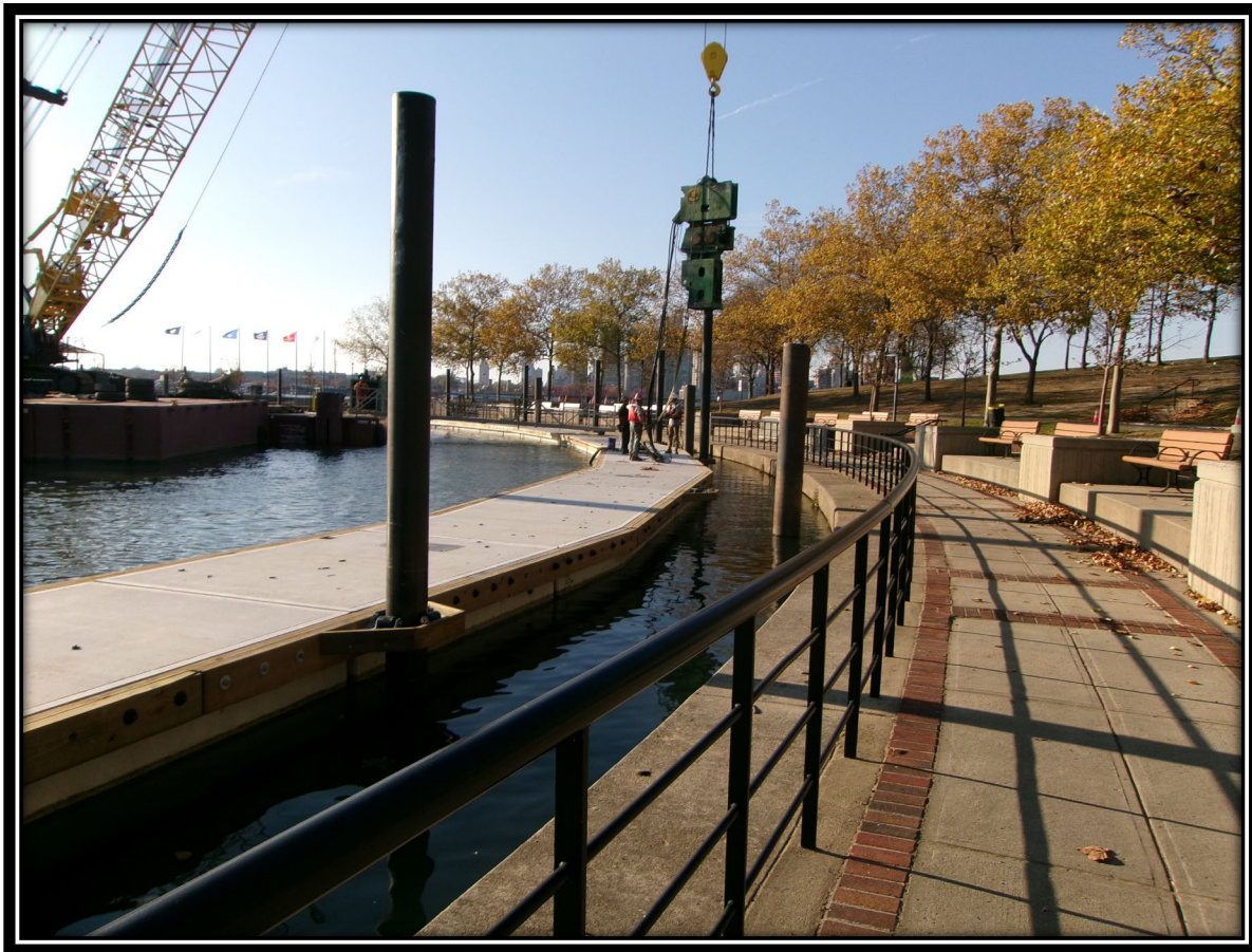
Figure: 1 – Install of pile guide and pile at the northern side of the marina
