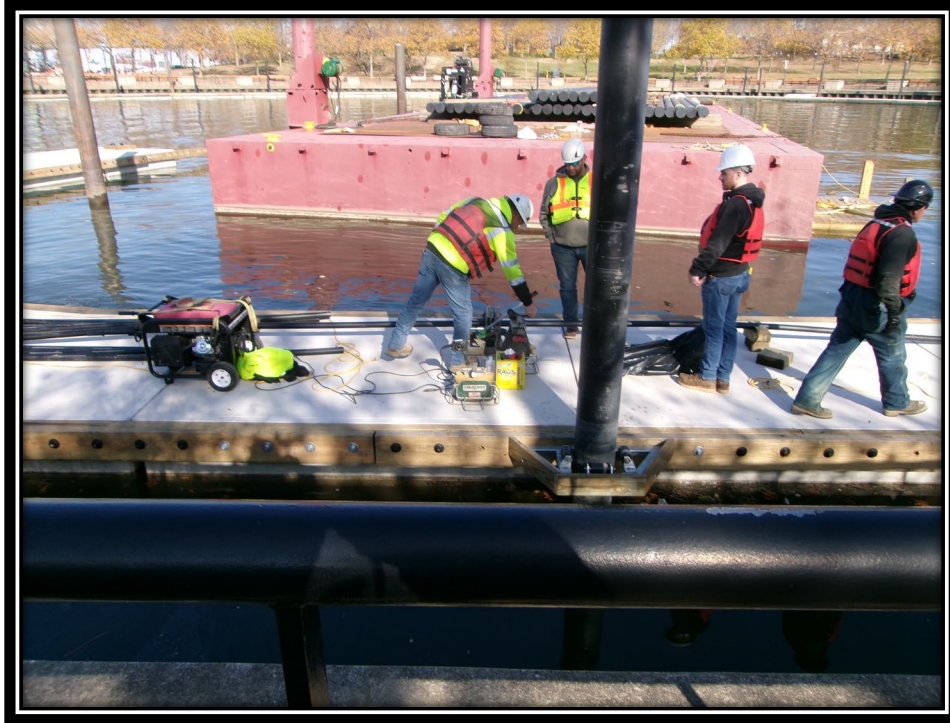
Figure: 2 – Installation of 2” PVC water service along the newly installed circular concrete floating dock system on the southern side of the marina
