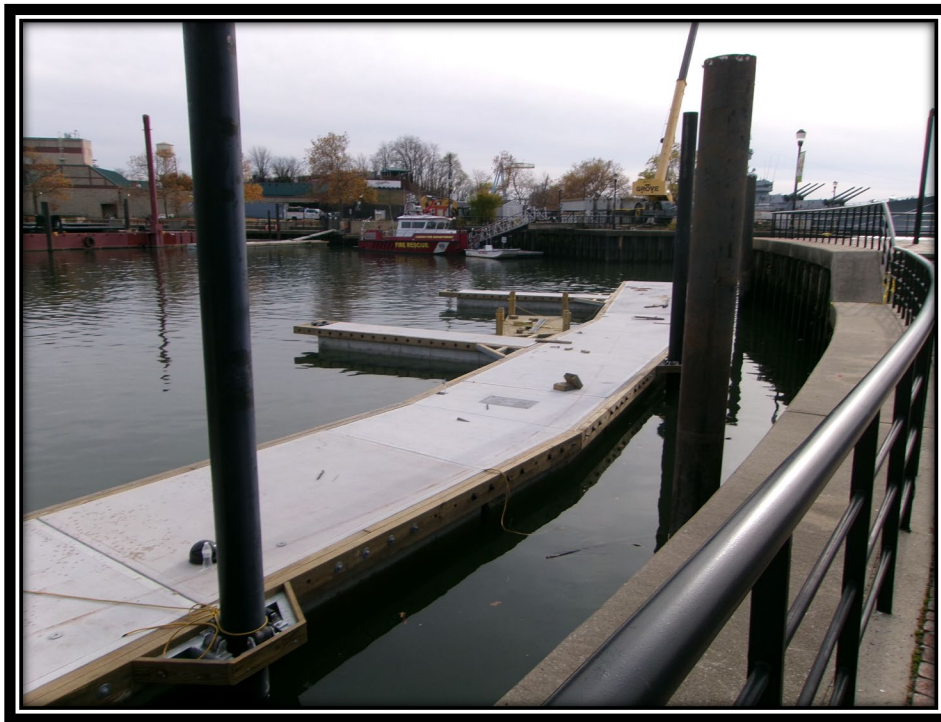
Figure: 3 – Installation of concrete floating finger piers at the far northern end of the marina
